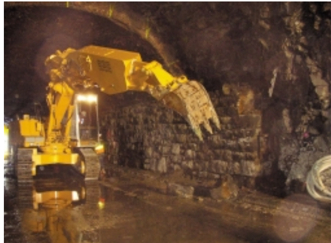
Liebherr excavator fitted with side bucket used to rip off old brick lining
